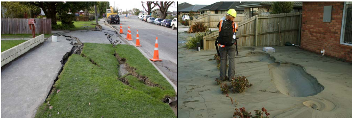
Figure 2: Examples of lateral spreading causing large cracks (left) and liquefaction (right)
