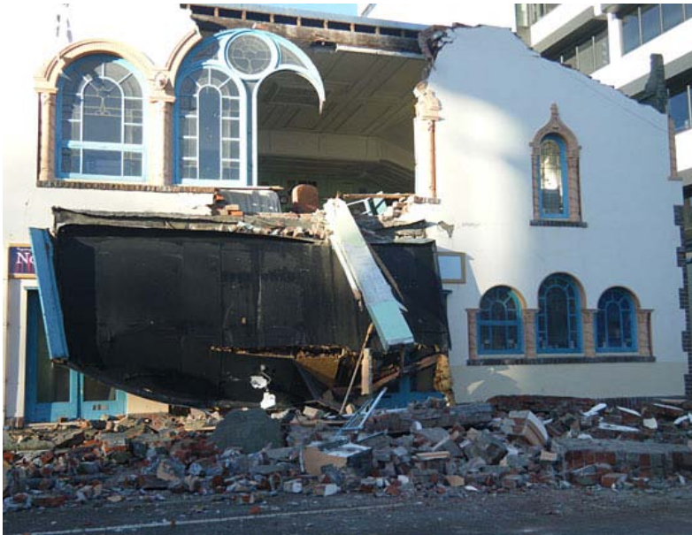
Figure 3: The Repertory Theatre - an example of damage to historic buildings in Central Christchurch (photo source: www.stuff.co.nz).
