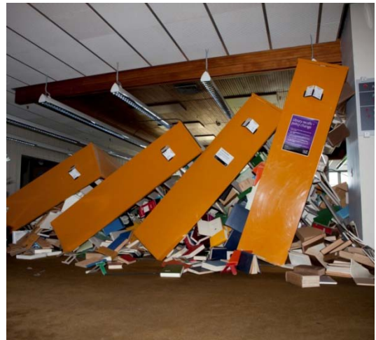
Figure 16: Collapsed library shelving created a real life-safety hazard.
